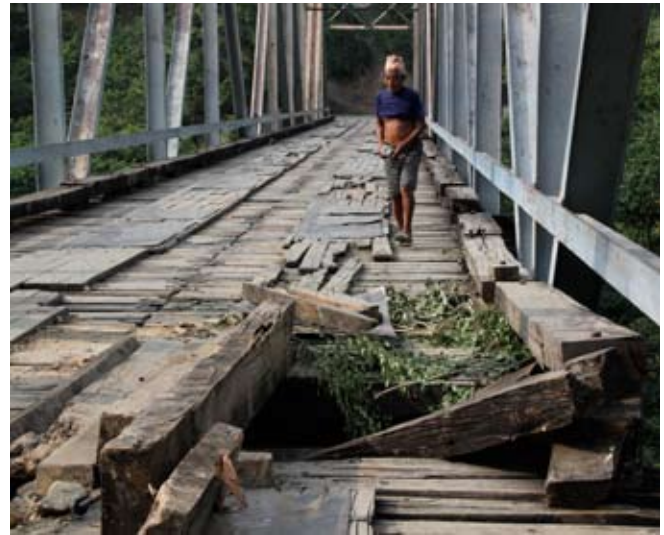
Big hole in Godavari bridge.
